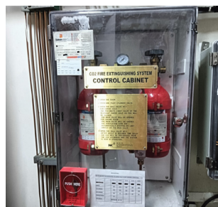
Fixed fire extinguishing systems (CO 2 , FM-200, NOVEC 1230, Water Mist)
