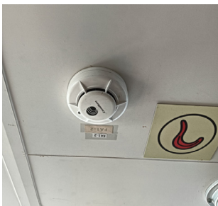
Fire detection systems (fixed & portable)
