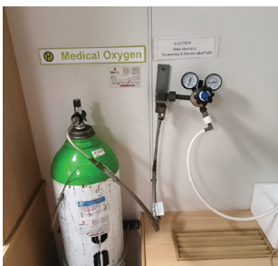
Medical oxygen systems (40L/200 bar hospital sets)
