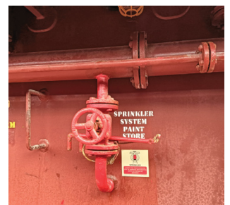
Sprinkler and clean agent systems
